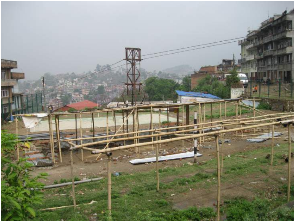
Figure 4.4: A safe space in one of the case study wards in Kirtipur where bamboo framed shelters were constructed following the earthquake.
