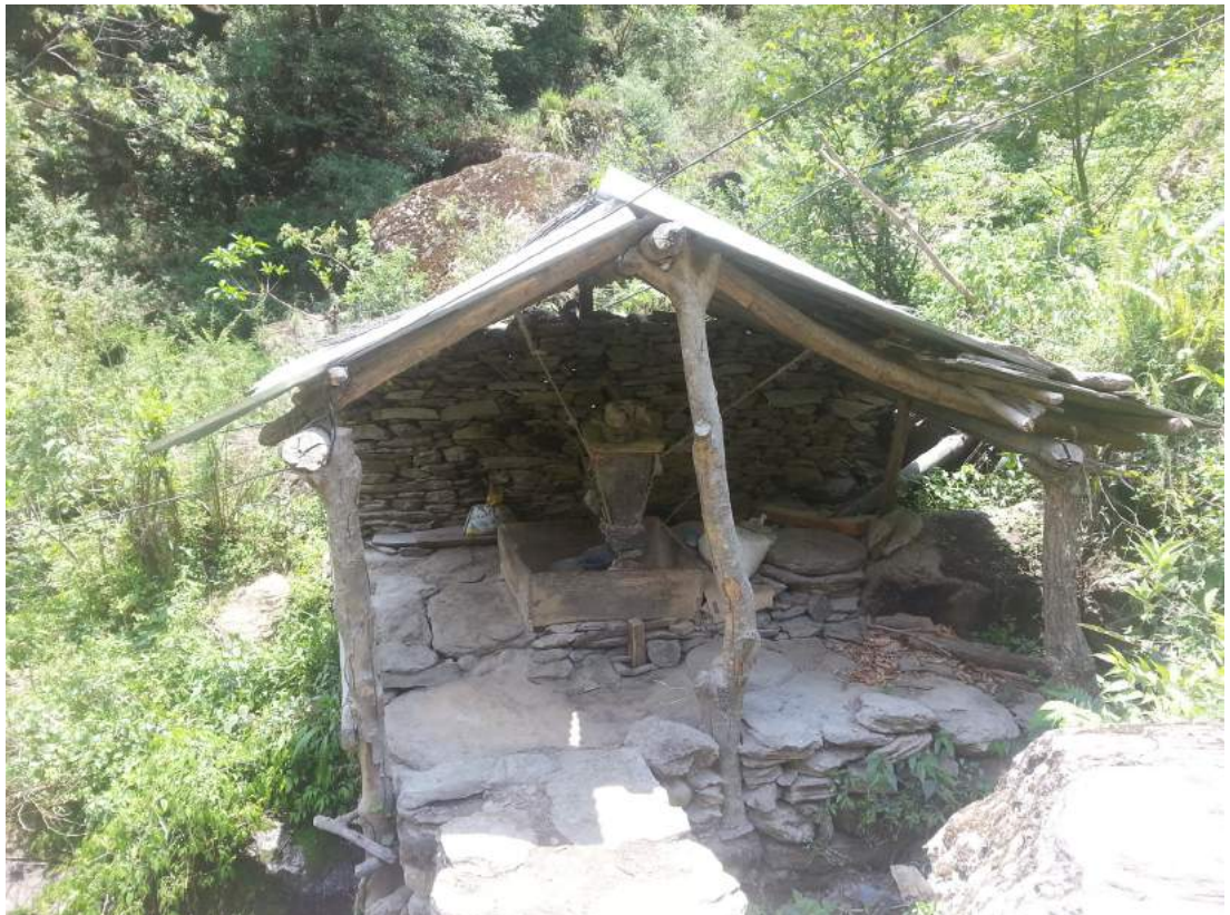
Figure 4.1: A water-powered mill or pani-ghatta in Dolakha District damaged by the 2015 earthquakes.
